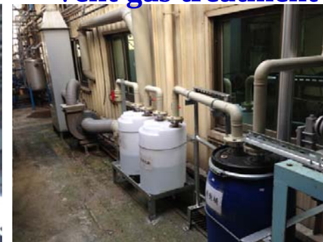
Vent gas treatment
